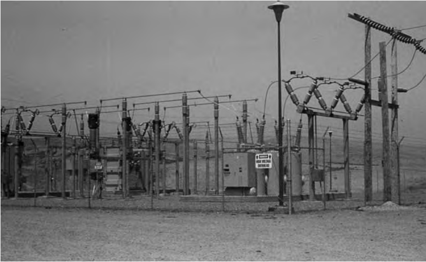
Figure 6.10 Distribution substation. (Courtesy of Marshal F. Merriam.)
