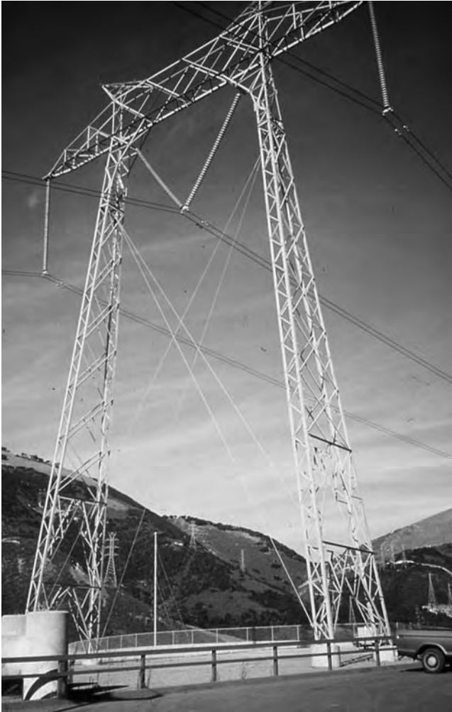
Figure 6.21 High-voltage transmission line. (Courtesy of Gene Rochlin.)
